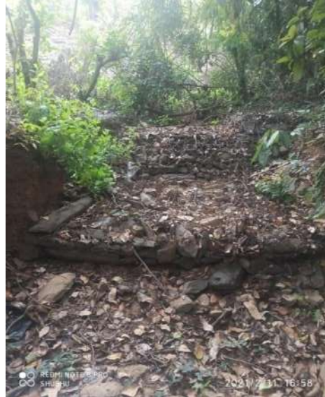
Gabbion check dam
